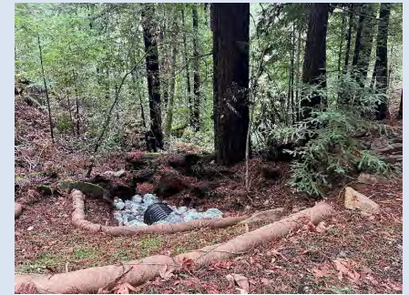
Figure 1A Rock dissipator and erosion control. Native duff covers all bare soil and erosion control seed has started to germinate.
