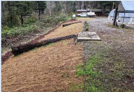
Figure 2: The slope was laid back to match the natural slope while supporting the road. Two log structures create habitat and protect the infrastructure during large storm events. Over 200 plants will be installed in Spring 2024.
